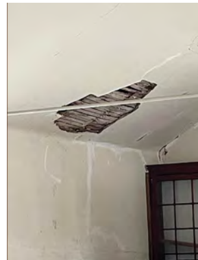
PORTION OF FAILING CEILING
